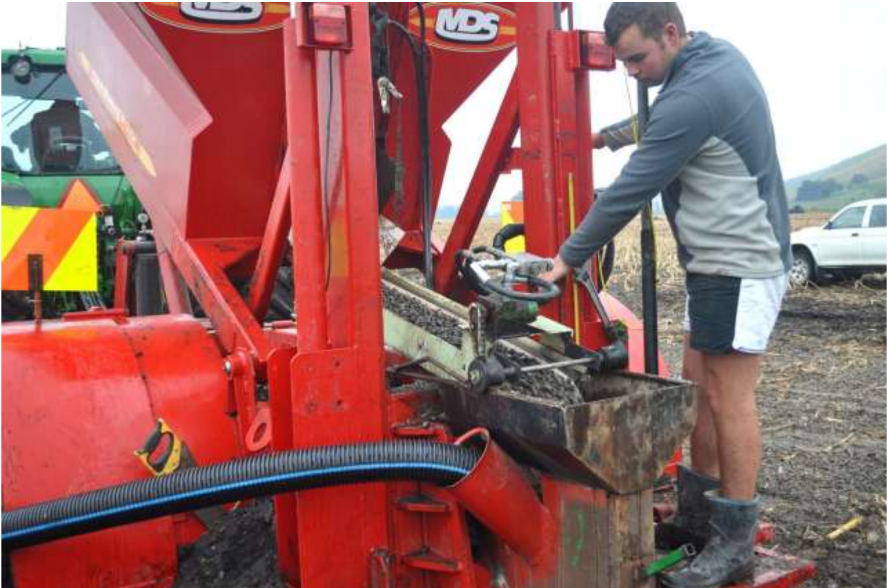
Figure 3 Drain pipe and gravel being fed into the machine - leg depth controlled by tractor GPS
