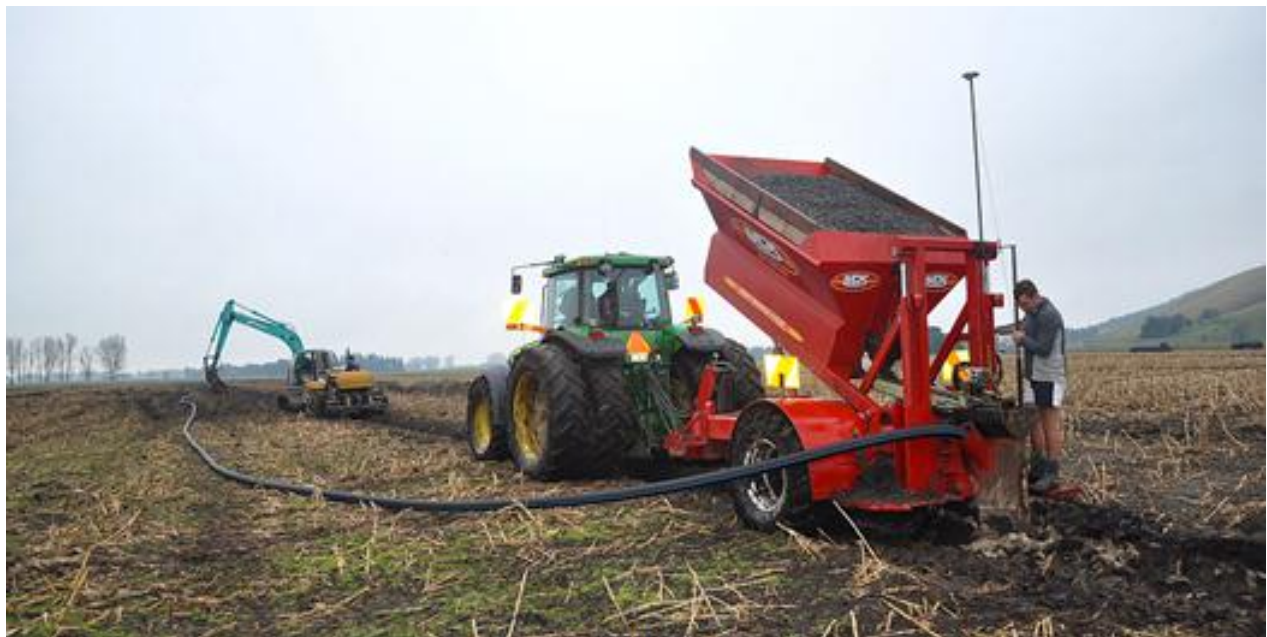
The drainlayer is able to work in poor conditions, all depth and grade controlled by GPS and software (Duke Dixon photo)
